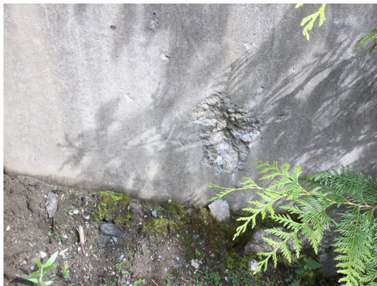
Minor damage noted to both ballast walls
